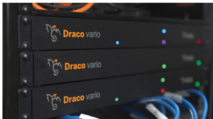
Server rack with KVM matrix switches
