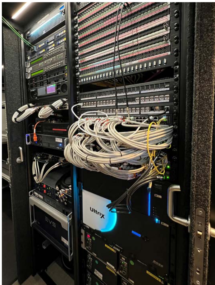
Space-saving accommodation of the KVM in the central equipment room
